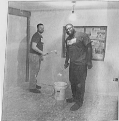
GCI employees Kelly Hall, left, and Ricky Colbert help apply primer to newly installed sheetrock at the Ketchikan Youth Initiatives facility on Park Avenue on Wednesday during a United Way of Southeast Alaska "Day of Caring" event.
